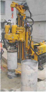
Geo-Bohrtechnik using a HBR 203 to drill 406mm-diameter micropiles to 15m depth in an existing building in Blaustein, Germany
