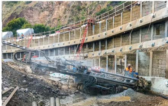
A Hütte Bohrtechnik rig was used during slope stabilisation work on Highway 1 in California after heavy rain caused mudslides
